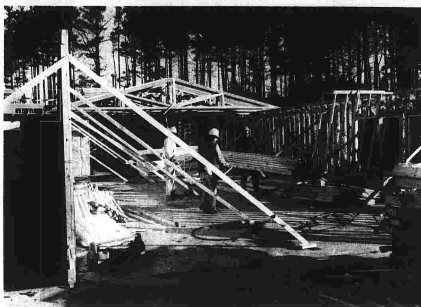
New roof trusses were in place this morning at the prefabricated student center at Manchester Community College. The trusses collapsed Wednesday afternoon when accidentally struck by a crane, injuring one construction worker.
